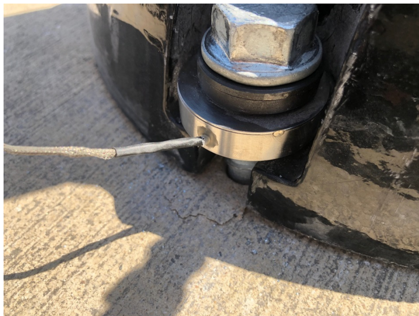
Figure 2 - Loss of Embedment at Load Cell
