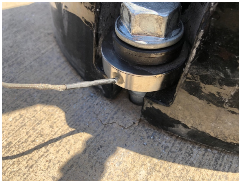
Figure 2 - Loss of Embedment at Load Cell
