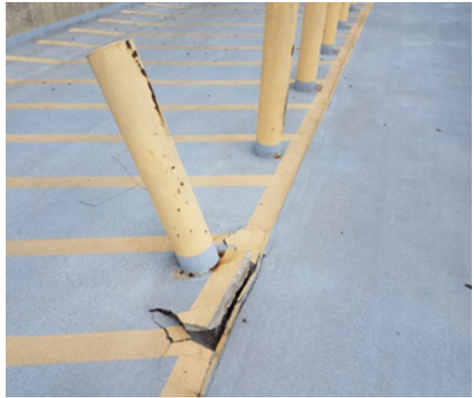
Figure 5 - Common Concrete Damage
